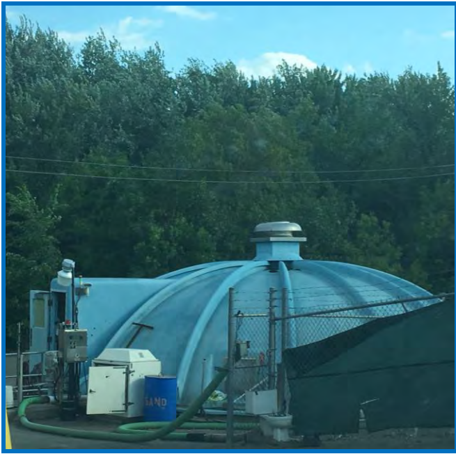
Brokaw Water Treatment Facility Source: NCWRPC, 2018
