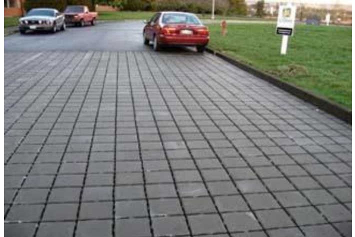
Permeable pavement reduces runoff. Source: epa.gov/green-infrastructure
