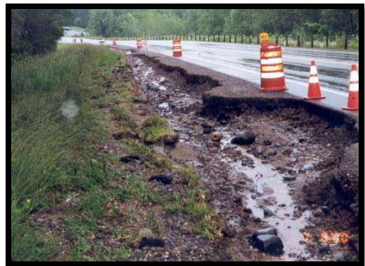
Hwy Flood Damage, Forest Co.
