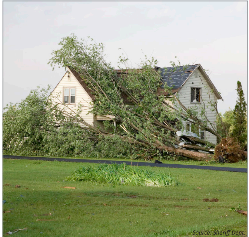
Storm damage to a house from a downed tree.
