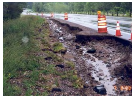
Flood Damage. US Hwy 8
