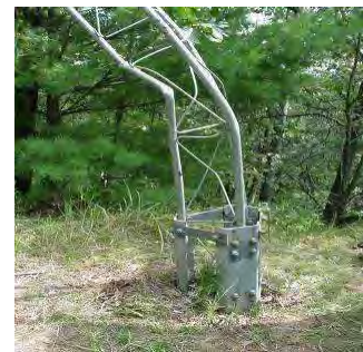
Wind Damage - Com. Tower
