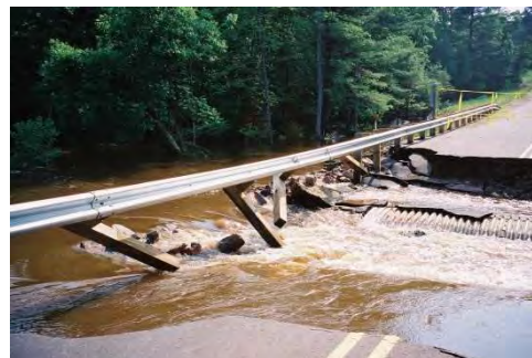
Adams County Highway Washout
