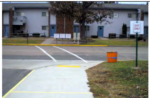
Barrier free sidewalk has no curb ramp across the street at the apartment complex.
