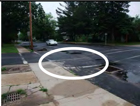
How do you cross when it rains? Crosswalk under water during a rain event.
