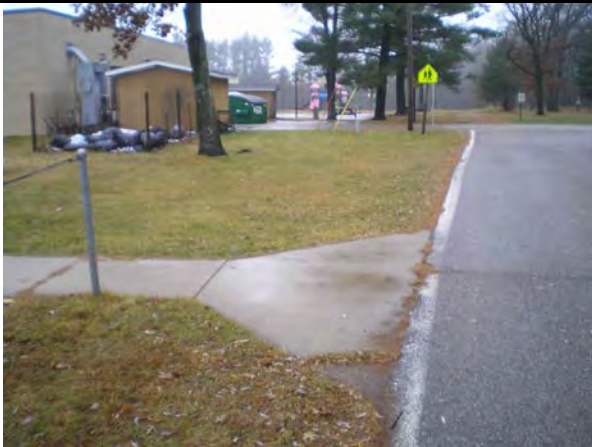
Pedestrians do not have an area to continue walking on. No crosswalk exists.
