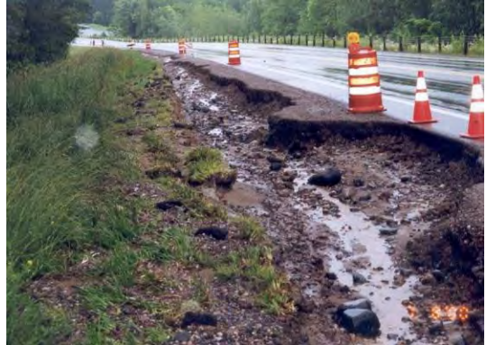
Hwy Flood Damage, Forest Co.
