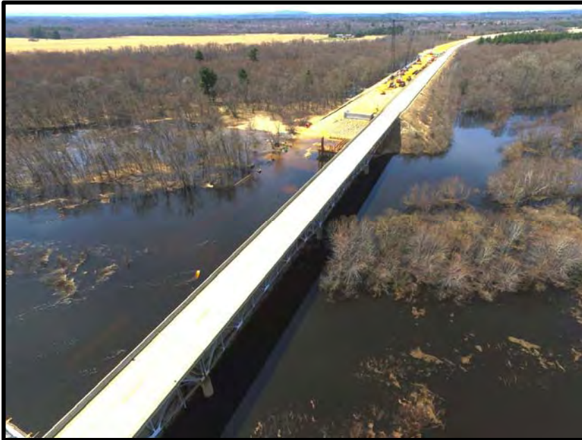
Excessive flooding can disrupt road construction projects, such as the construction project for the State Highway 82 Bridge that connects Adams County and Juneau County.
