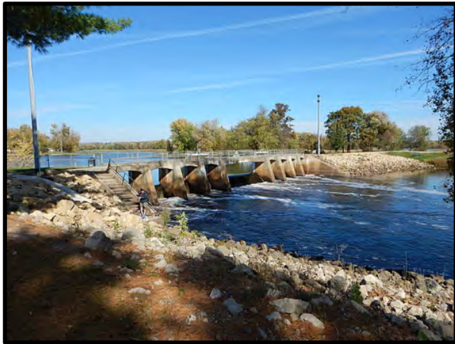
Dams like the New Lisbon Dam pictured above should be inspected every two years. Image source: Wisconsin River Trips
