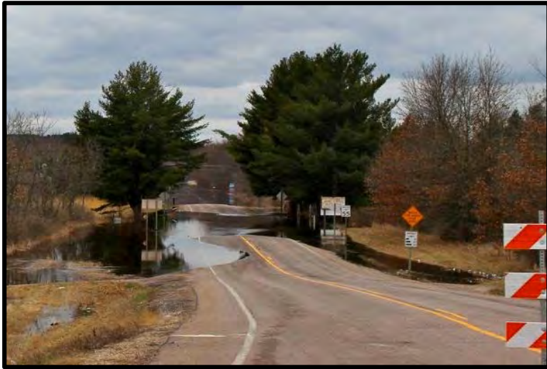
Flooding of the County Highway HH - State Highway 82 intersection in the Town of Kildare.
