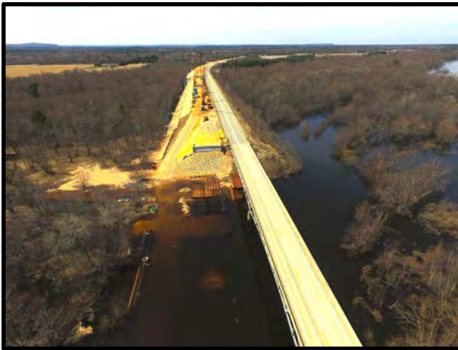
Construction on the State Highway 82 bridge was delayed in 2018 due to excessive flooding. Image source: Rocky Gilner
