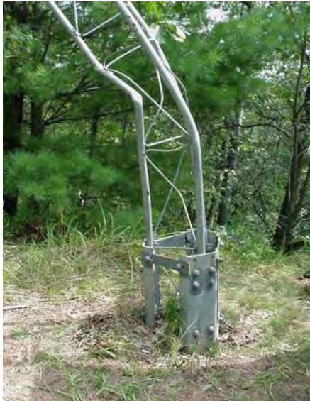
Wind Damage - Communication Tower
