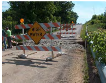
New Haven Flood Damage
