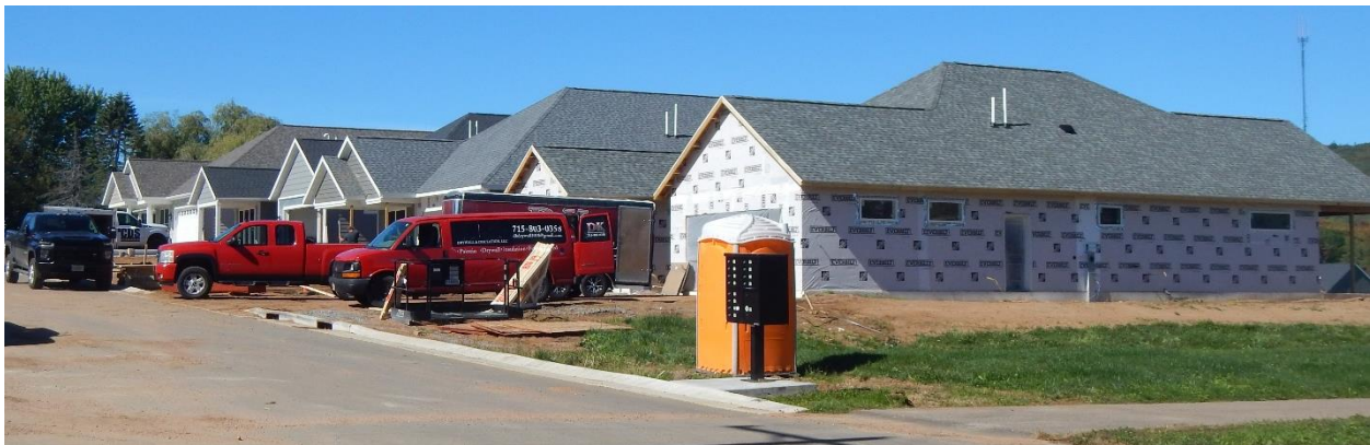
Above: Slab-on-grade homes are increasing in popularity since they reduce construction and energy costs and allow for barrier-free, ADA-accessible living as the region's population ages.
