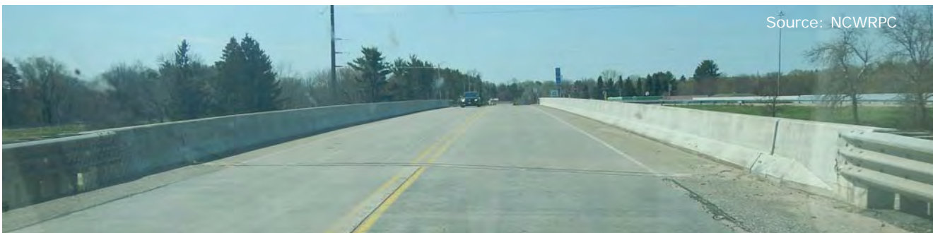
A bridge without railings
